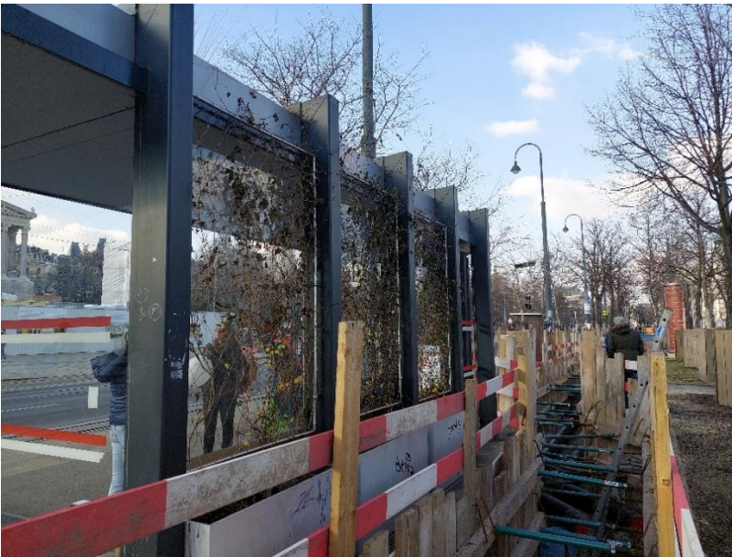
Figure 2: Construction site of a climate-adapted bus stop at Parliament. Image Credit: Wiener Linien.
