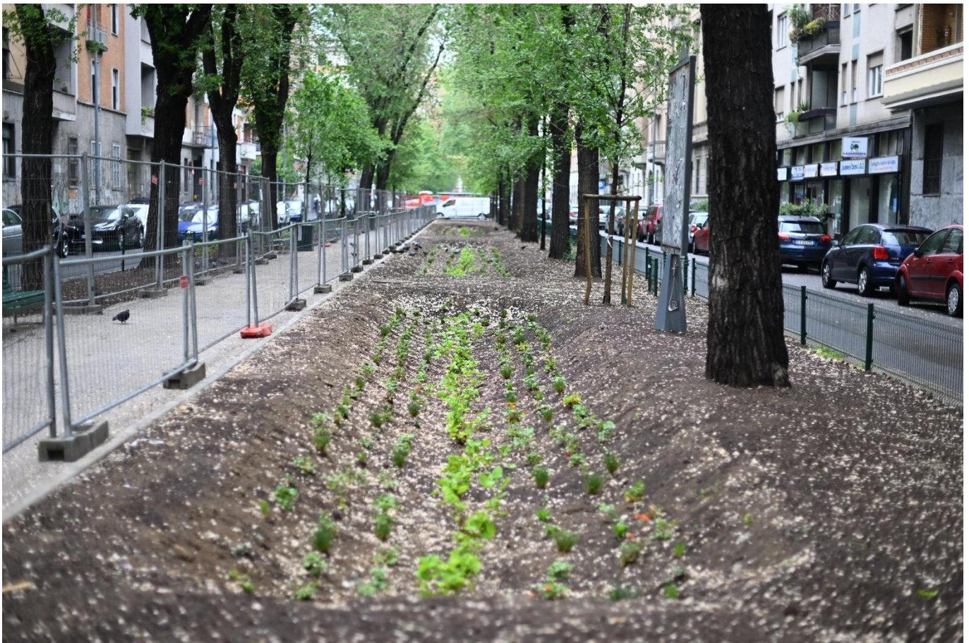
Figure 1: The first sustainable urban drainage system of Milan. Image Credit: Comune di Milano.
