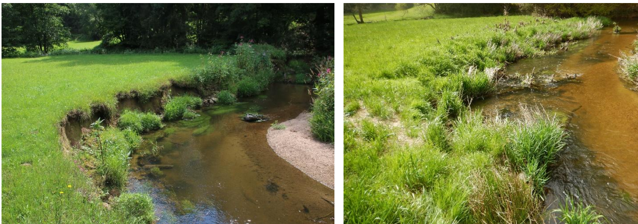
Figure 1: River bend before (left) and after (right) river restoration. The project team flattened the eroding and collapsing riverbank providing stability and increasing floodplain connectivity. Deadwood and boulders provide shelter and habitat structures for aquatic organisms as well as increase hydraulic roughness of the formerly monotonous river channel. Image Credit: © Marco Denic, Landschaftspflegeverband Passau.
