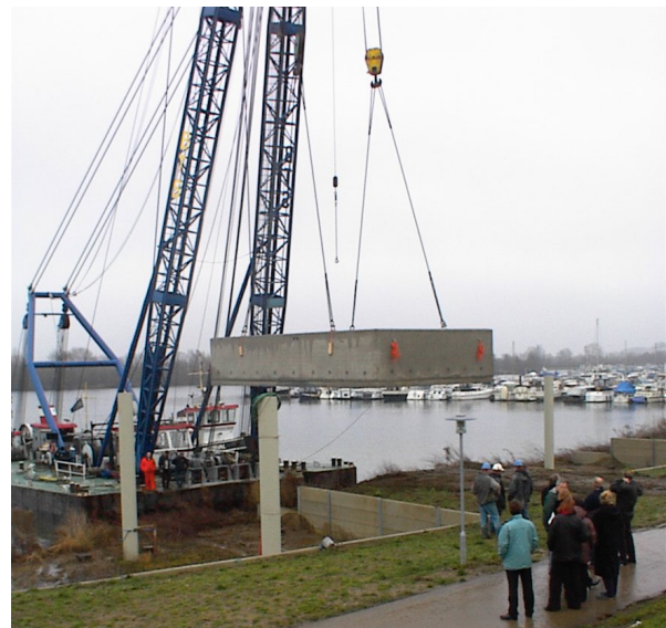
A concrete hull is hoisted from the water into the dock of a amphibious home.
