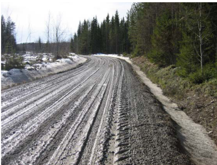
Figure 1: Surface frost heave problems on a gravel road
