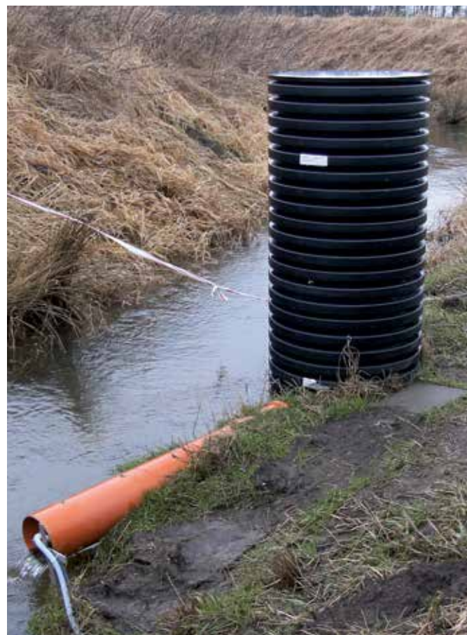
Figure 2: 'Controlled drainage' unit, © Tilo Hartwig
