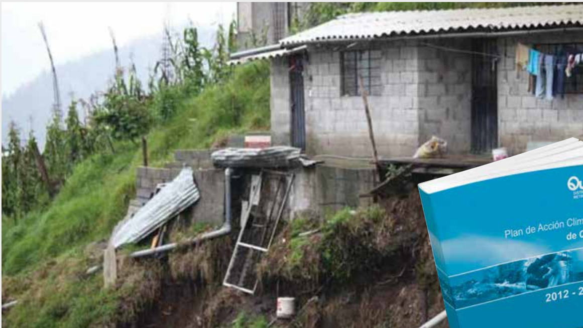
Inadequate housing on a steep slope in Quito. © Agencia Pública de Noticias de Quito
